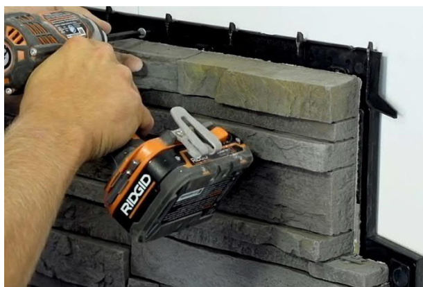
Figure 2. A typical “beonstone” installation
